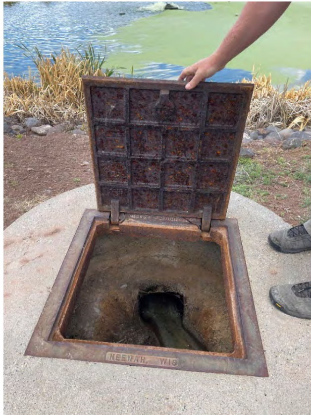
Figure 21. Cell No. 1 Influent Manhole
