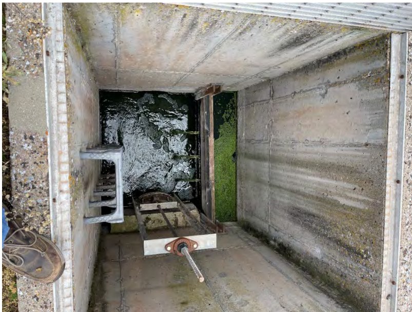
Figure 28. Diversion structure condition
