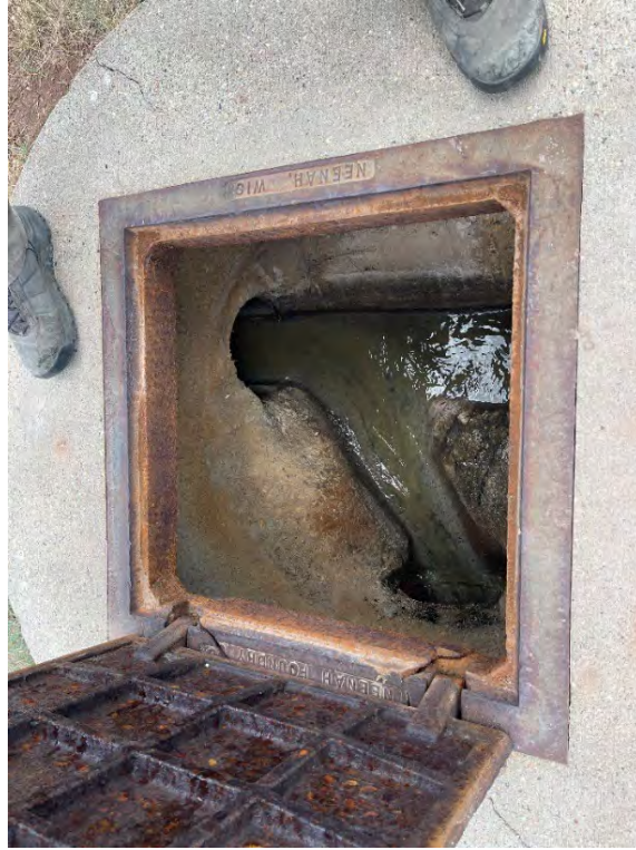
Figure 20. Cell No. 2 Influent Manhole
