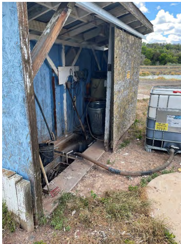
Figure 16. Influent/Headworks Building Interior
