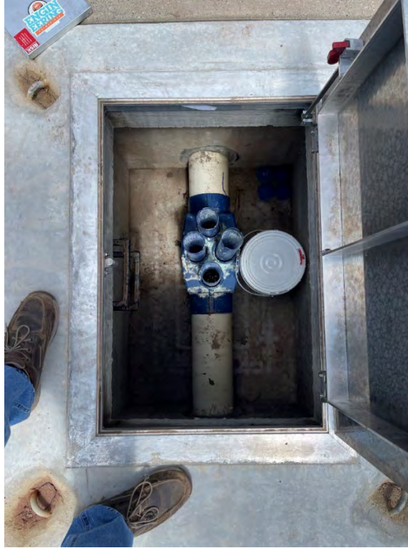
Figure 32. De-Chlorination Chamber condition
