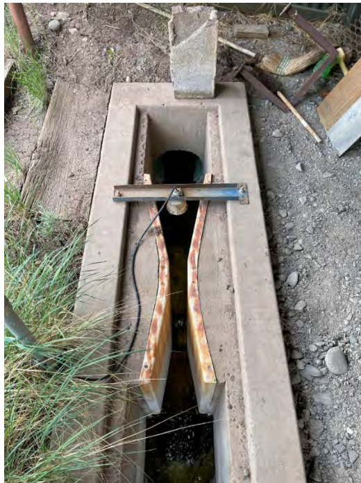
Figure 33. Discharge Flume condition
