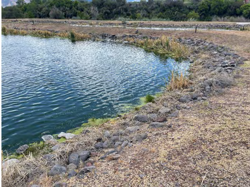
Figure 23. Cell No. 2 Berm Condition
