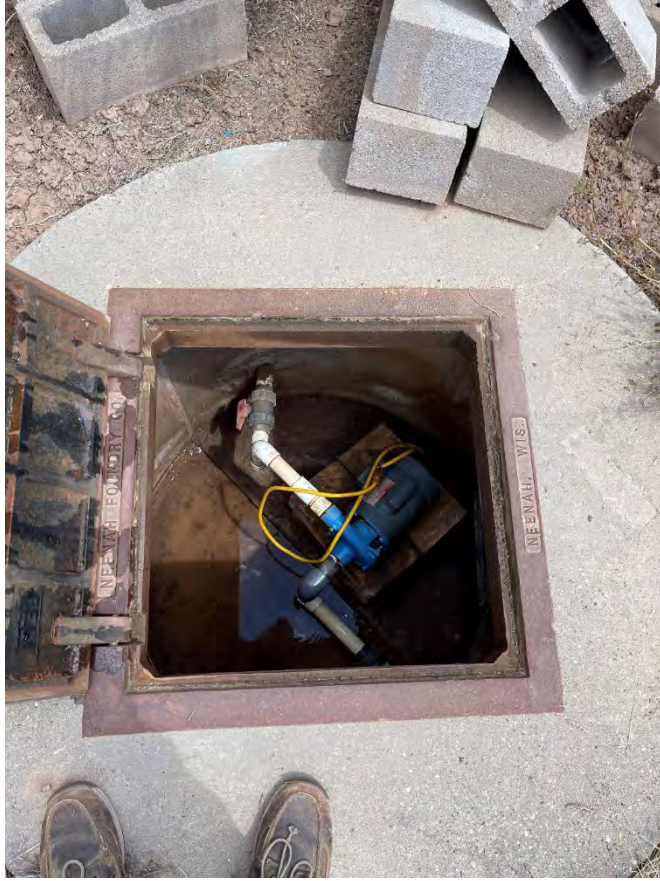
Figure 30. Chlorine Recirculation Pump structure condition
