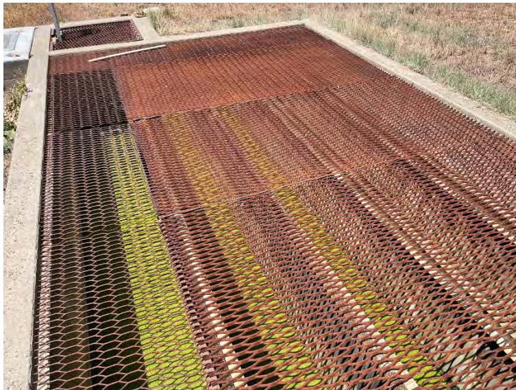
Figure 31. Chlorine Contact Chamber grating condition
