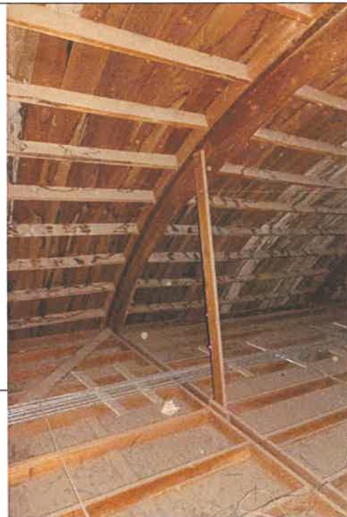
32: Visible water damage on decking and framing.
