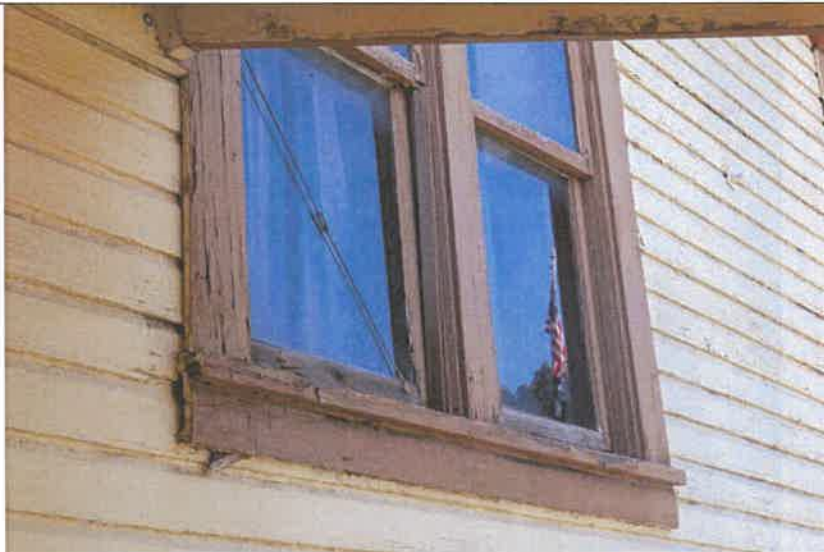
8: West façade – east double hung window paint peeling and sill degradation.
