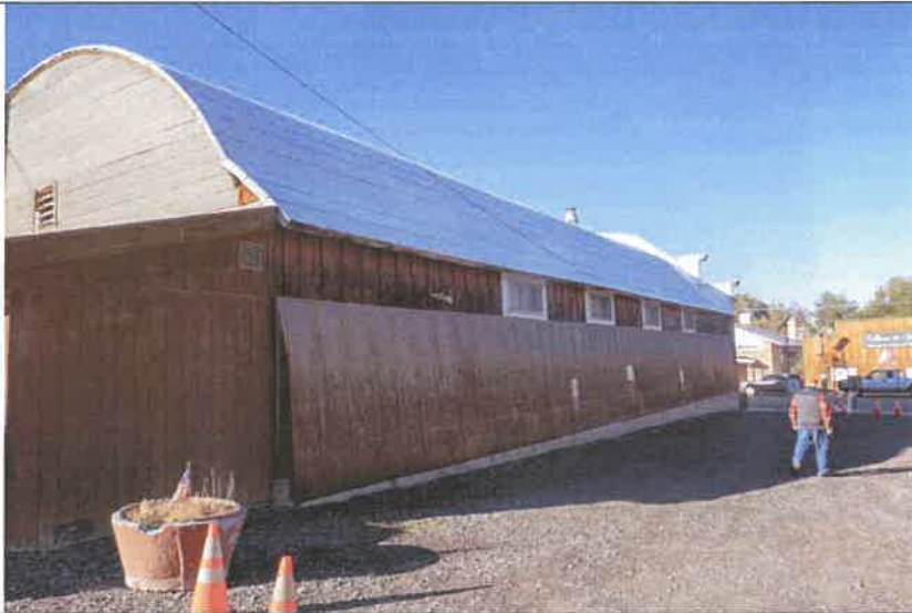
3: North Elevation: the clerestory windows were originally the only portion covered by the secondary roof slope overhang.
