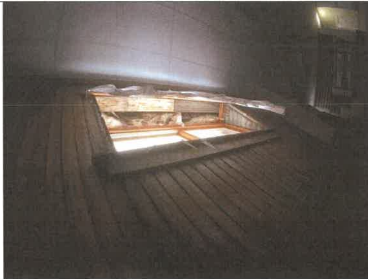
24: Assembly Hall 104 clerestory water damage.
