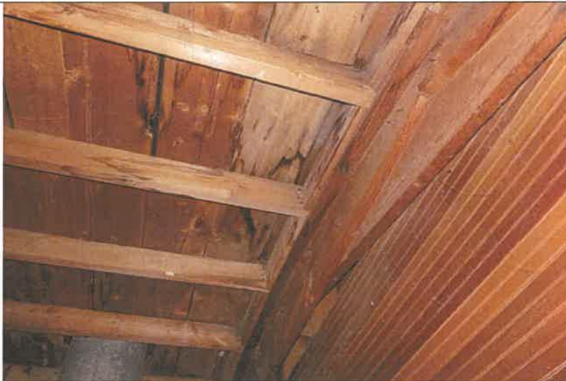
31: Framing at end walls showing deck water damage.
