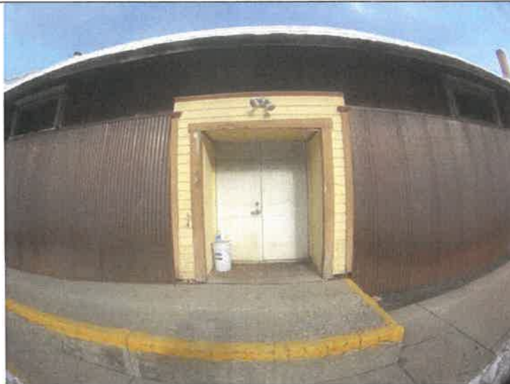
10: South Elevation entry with non ADA compliant ramp.
