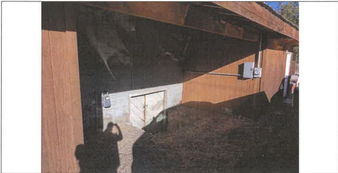
11: East Elevation basement entry, gas meter and electrical panel and meter.
