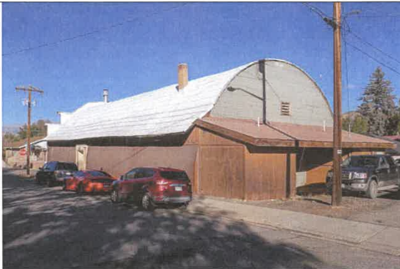
4: South Elevation: the south clerestory overhang extends farther than the north and is visibly bowed.
